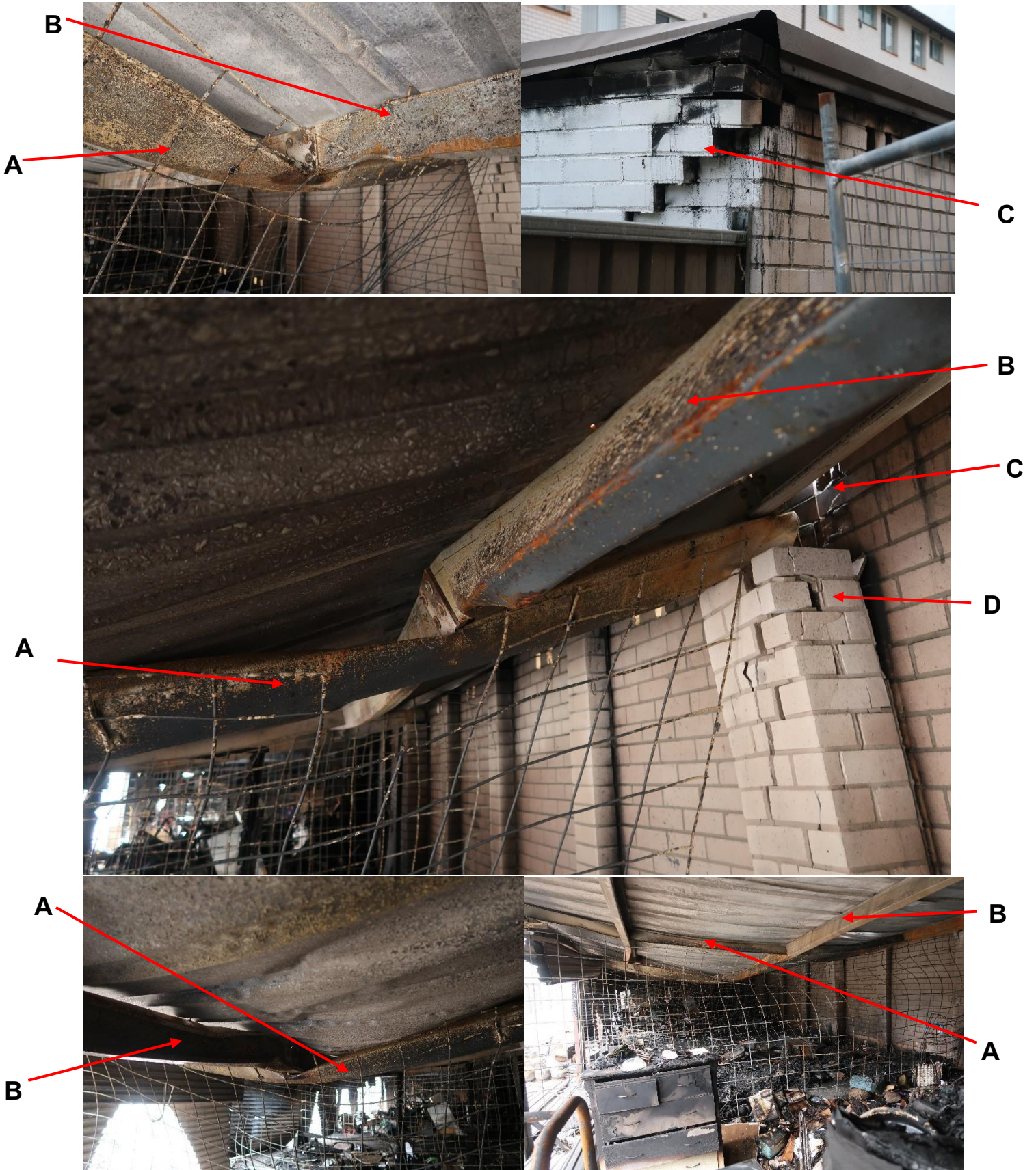
Extreme heat due to the involvement of volatile materials, including polyurethane foam-based furniture, caused structural steel to soften and weaken, becoming displaced. In the above views, the steel A beams and B purlins supporting the roof initially expanded (pushing outwards) then sagged, causing steel to pull in. Displacement of the steel caused movement of the C upper brick walls and D brick support columns, creating openings (that could potentially fire to vent) and causing the walls to crack become unstable, presenting a collapse risk.
