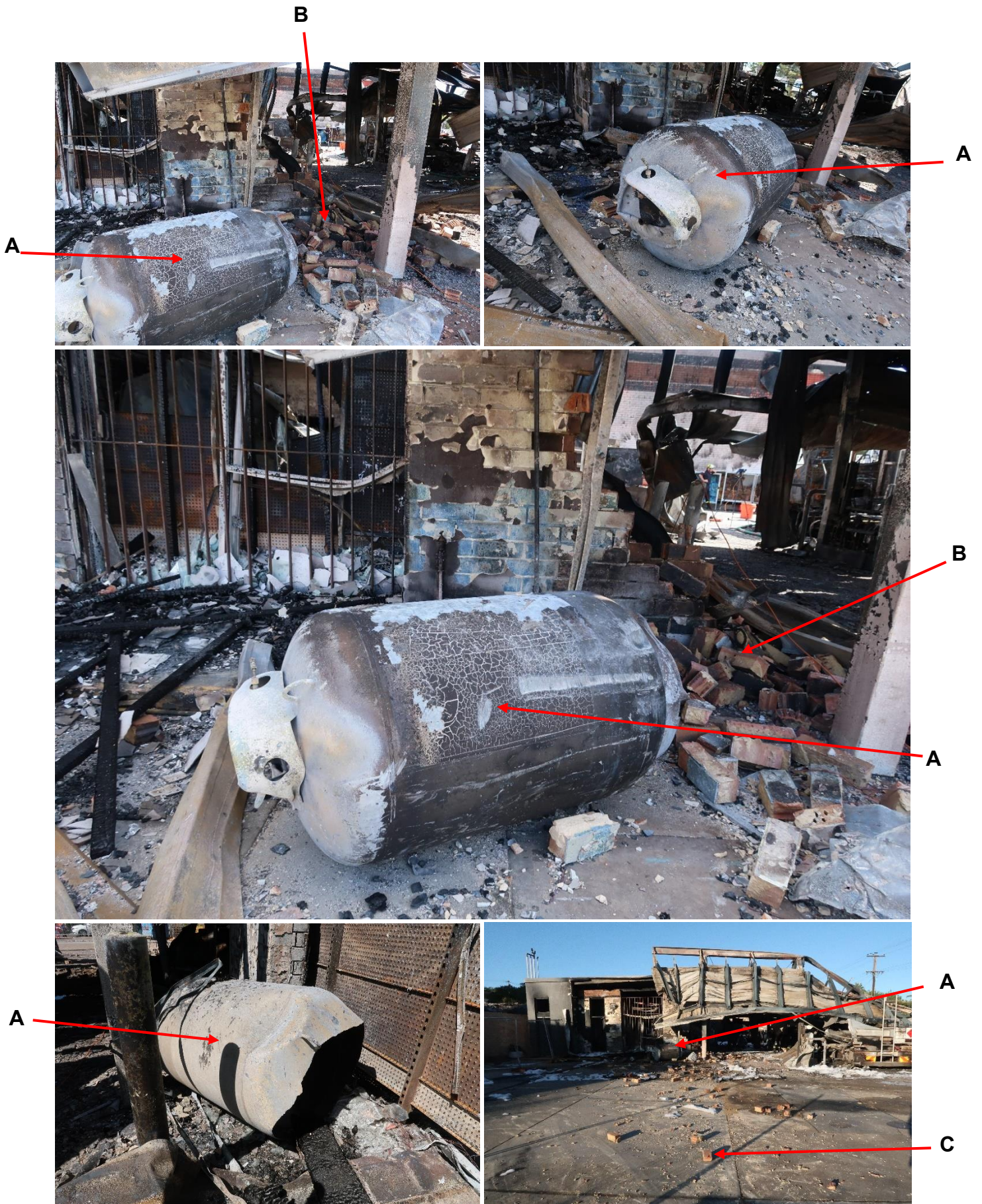
As a result of boiling liquid expanding vapour explosions (BLEVEs) of two 210 kg LPG cylinders, the cylinders became projectiles with sufficient force to breach the brick walls of the service station building. These views show where the two cylinders (A) came to rest after breaching the walls (B) and displacing brick debris 20 metres beyond the wall (C).
