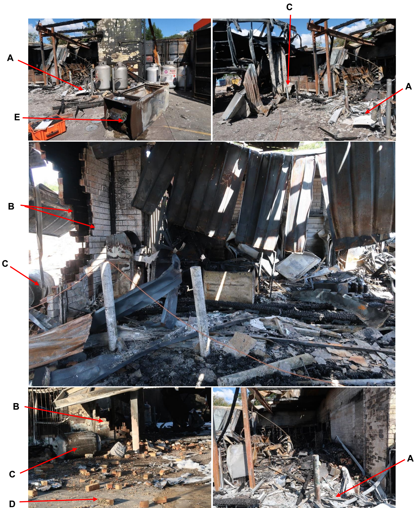
Boiling Liquid Expanding Vapour Explosions (BLEVEs) occurred involving two 210 kg LPG cylinders located at (A) the front of the service station building. The force of the explosion was so powerful one cylinder demolished (B) a double brick wall before (C) coming to rest after breaching the wall and (D) scattering debris. The shockwave associated with the BLEVE of a second cylinder caused the displacement of (E) an ice making machine. Firefighters used distance and shielding to protect against the effects of the BLEVEs.
